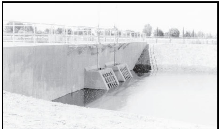
Upstream side of dam showing manual sluice gates which are used when complete shut-off is desired.
